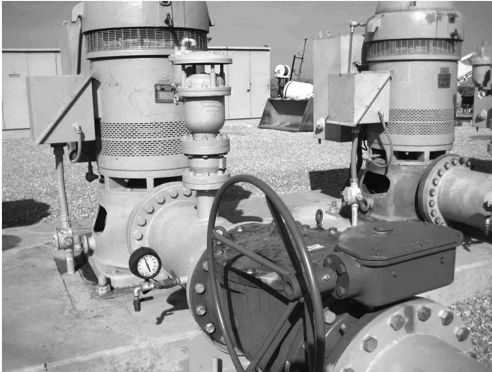
Figure 1-2 An air valve installed on the outlet of a pump and upstream of the check valve
